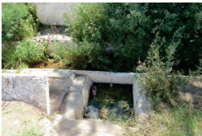
Fig. 4. Current condition of the Maylibay Irrigation Canal and its hydro posts.
